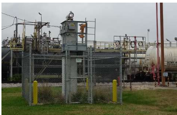
An OPSIS fence-line system installation.
